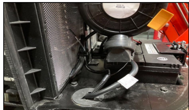
Fig. 13.9 (Coil Wires Behind Battery)
